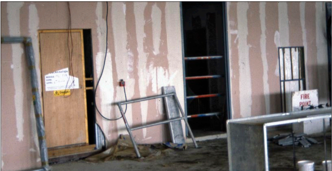
Figure 14 Plasterboard partitions such as this can form effective compartmentation. It is important that all gaps are filled in. In this case, there are holes in the top of the partition and service ducts in the side rooms that need to be sealed
